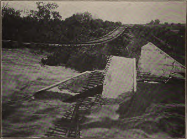
FIG. 31.—This wreck was caused by an insufficient bridge opening. A head of about seven feet was created and the excessive velocities undermined the piers though resting upon piles.
